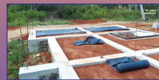
Construction of Transit Houses for pilgrims at Madhu Shrine, Mannar for SLR 401 million
