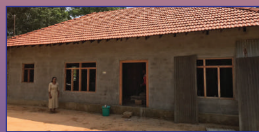
Construction of houses under Grama Shakthi and Model Village Housing Projects across Sri Lanka
